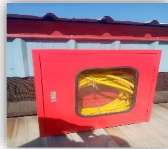
Water Hose Boxes fixed on roofs
