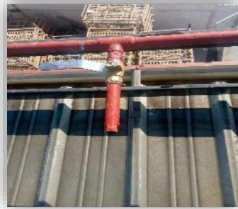
Water connections on the roof
