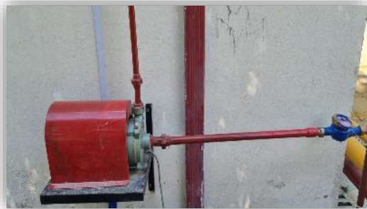
Water Pump for water points on the roof
